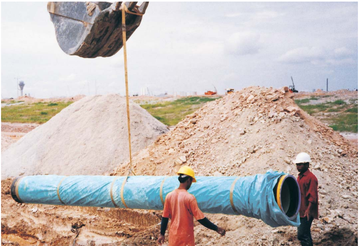
Sleeving pipe with Pentair Water Solutions’s POLYBOSS at Kuala Lumpur International Airport
